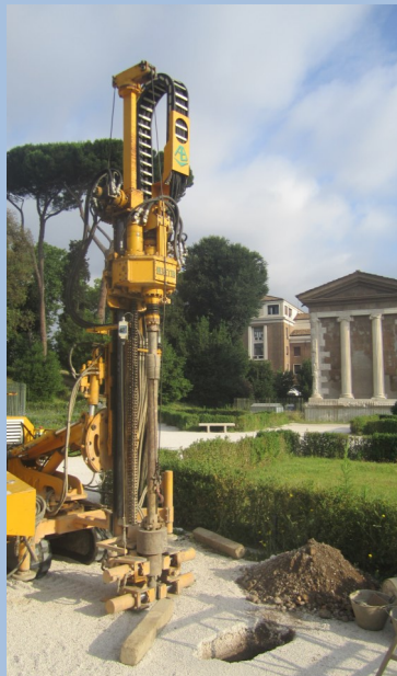
Drilling machinery during the production of a borehole behind the Temple of Portunus in the Forum Boarium.
